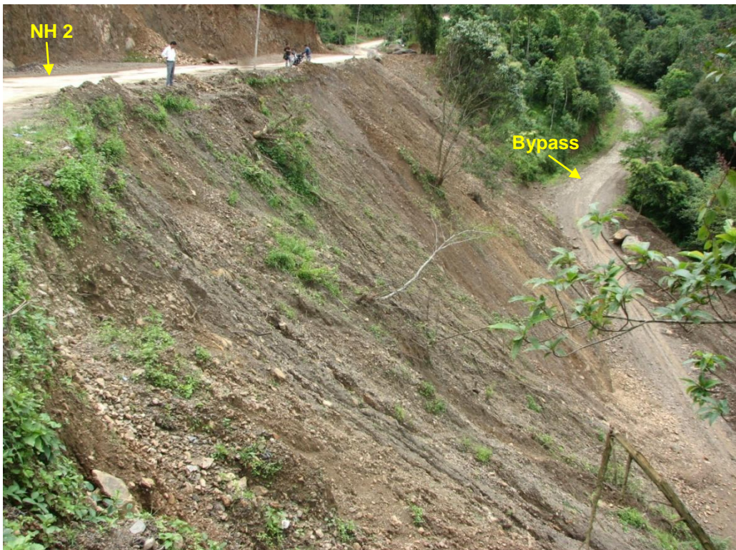
Plate 7.11b. Unstable steep slope between NH 2 and Bypass
