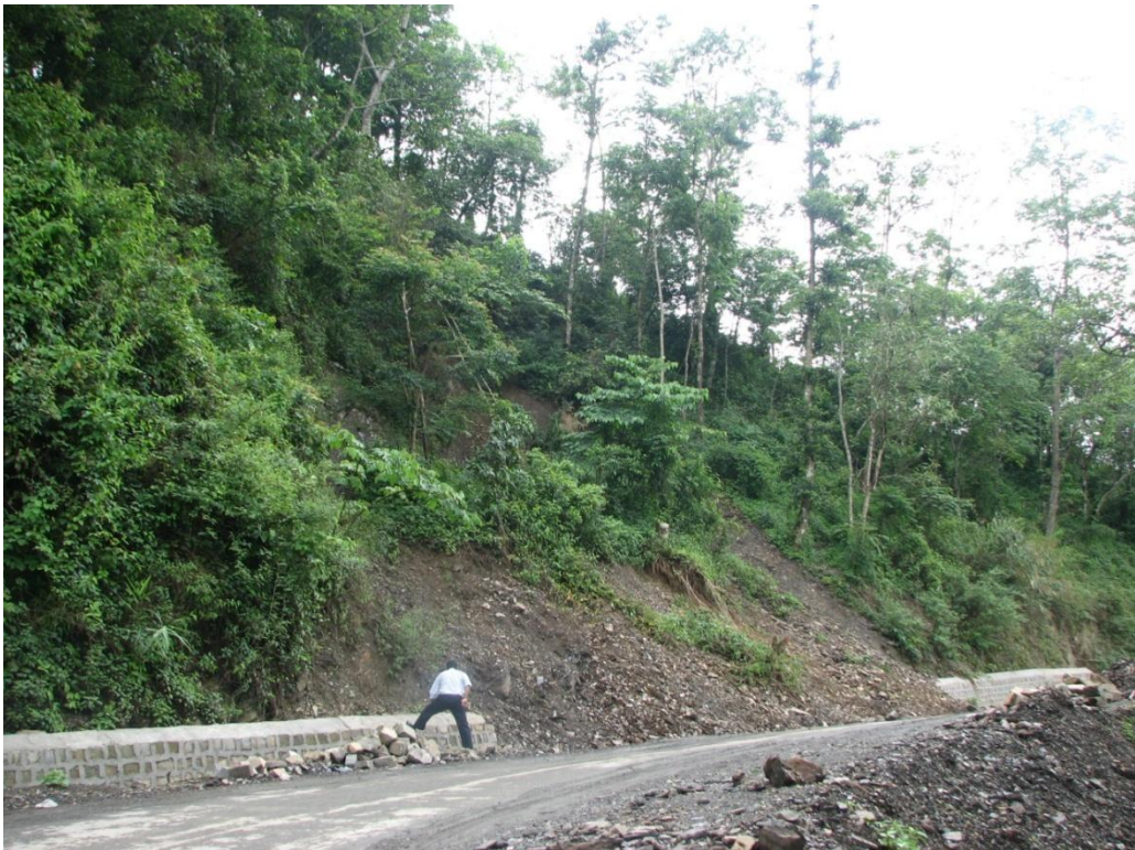
Plate 7.5b. Blocked roadside drain
