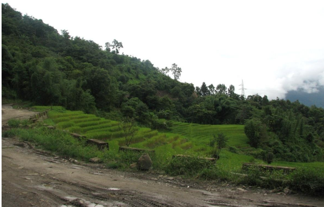
Plate 8.4. Damage of road due to terrace cultivation
