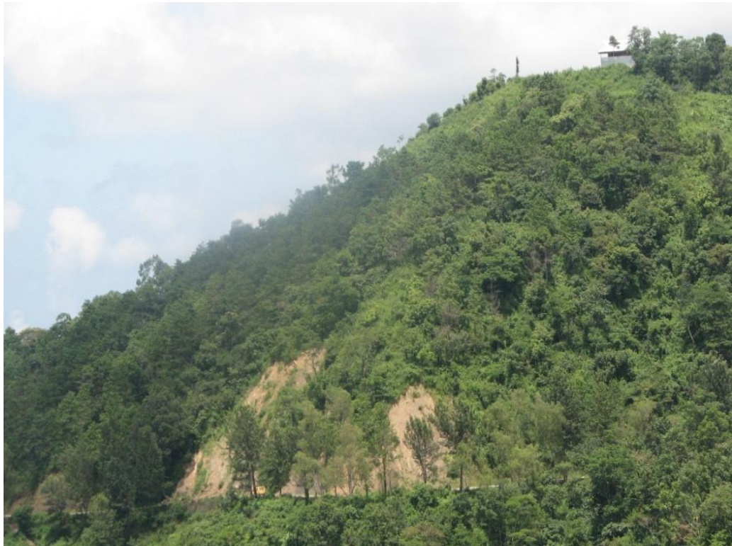
Plate 7.7a. View of debris slide scar
