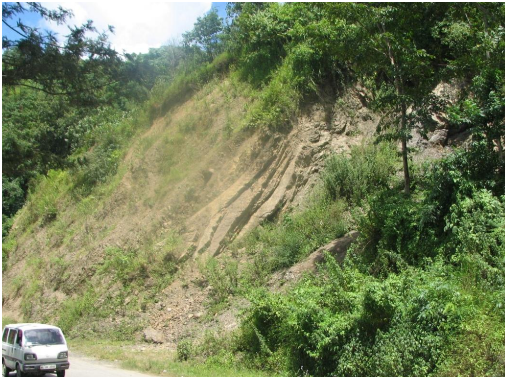
Plate 7.6b. Drainage blockage by debris
