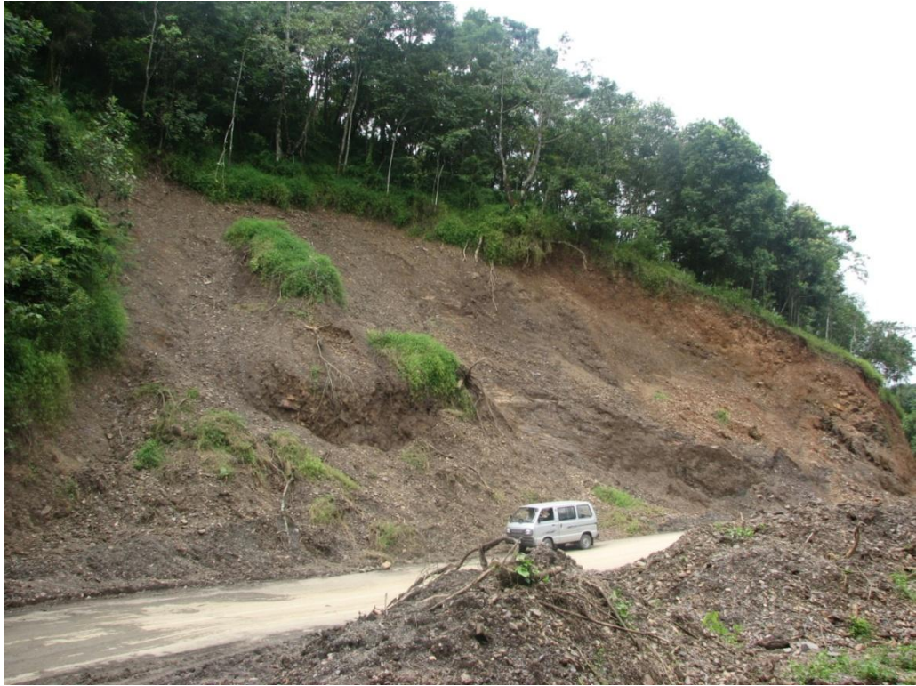
Plate 7.12a. Critical condition of slope
