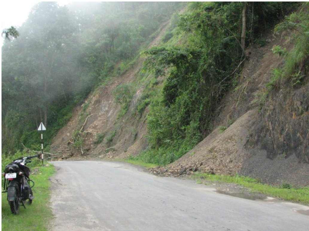
Plate 7.7b. Drain blocked by debris
