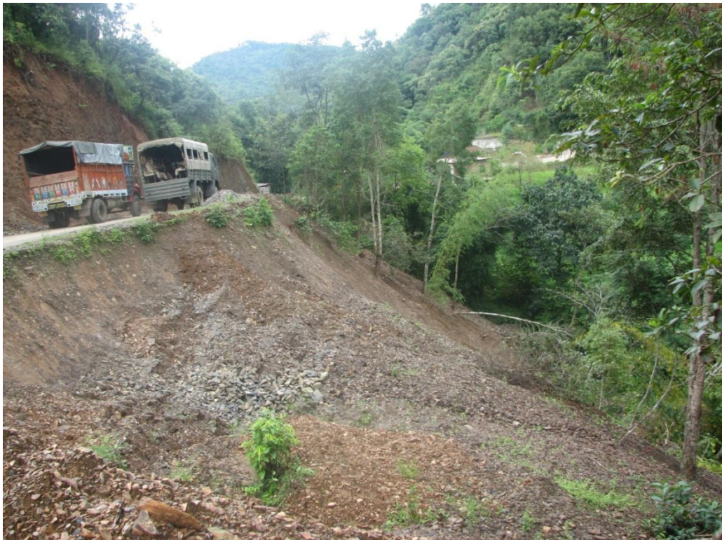
Plate 7.13b. Subsidence of portion of highway
