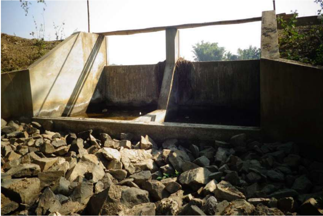
Plate 21: Water harvesting structure at Ranibheta, Titabor, Assam
