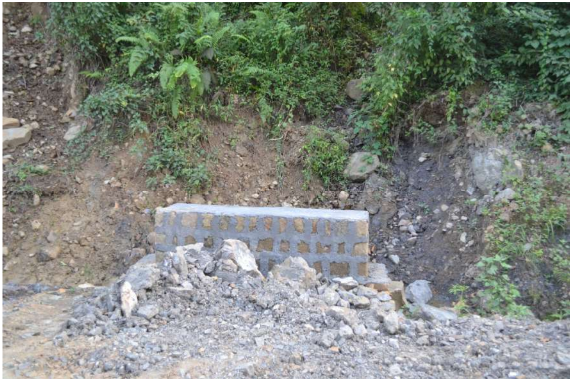
Plate 7.1.2.a Drains choked by debris
