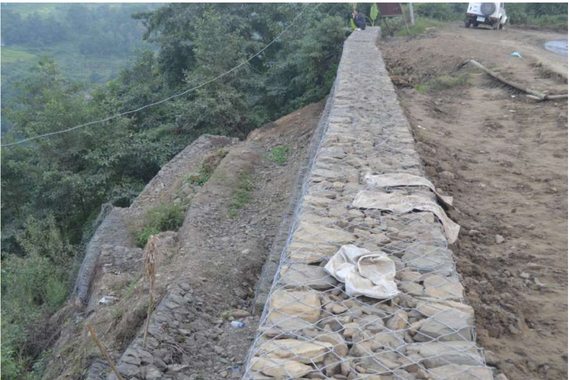
Plate 7.1.a Creeping indicated in man made structure
