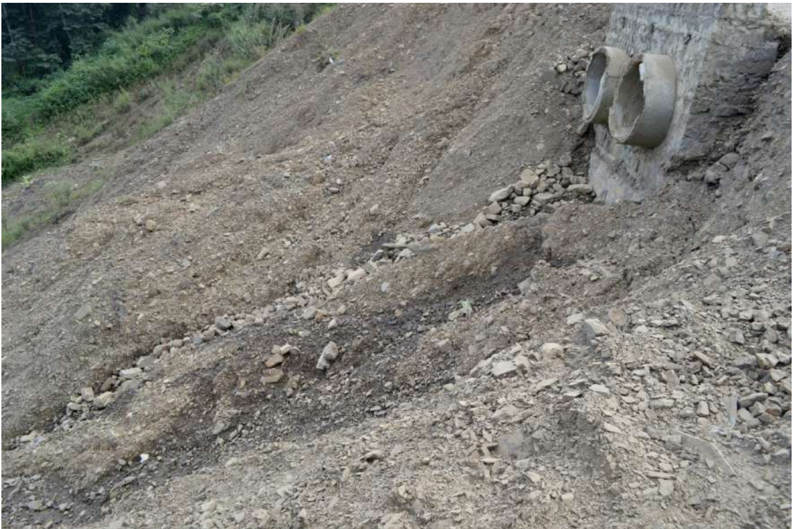
Plate 8.2 Water draining in an unstable area
