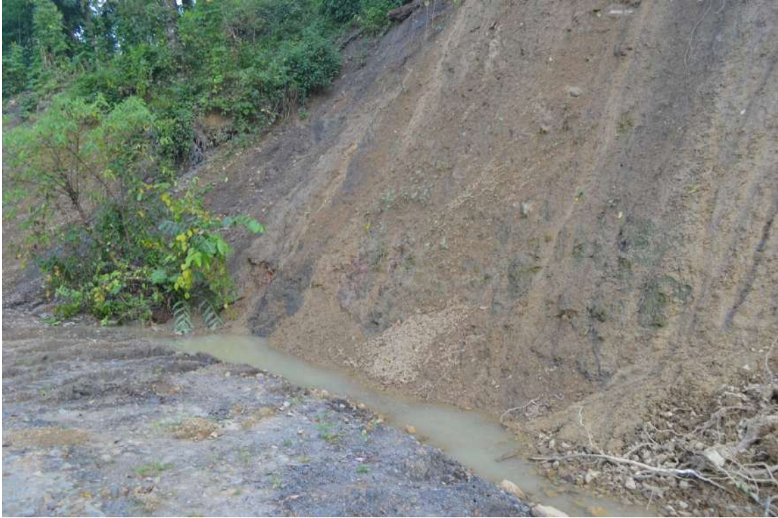
Plate 7.2.2.b Concentration of sub-surface water
