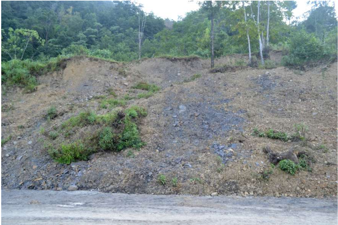
Plate 8.1.d Debris Slide along the Highway
