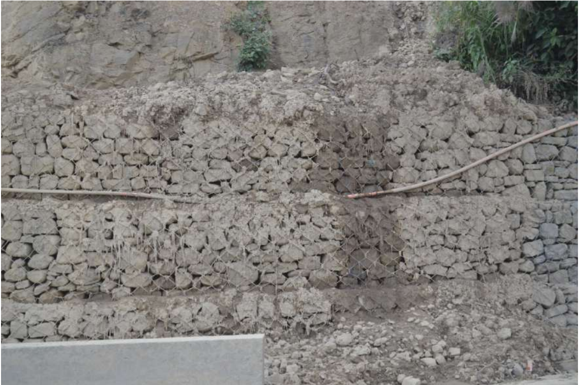
Plate7.1.2.b Water seepage from upper slope
