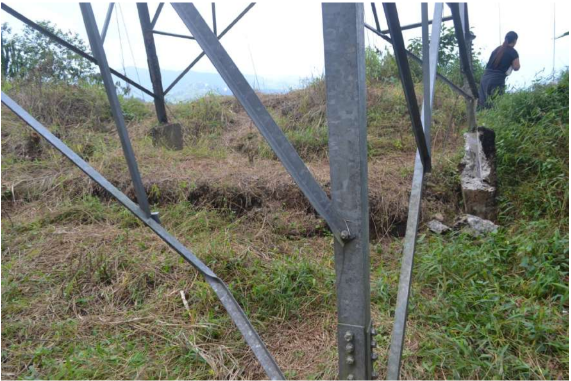
Plate 7.1.2.c Tilted High Tension Power Line
