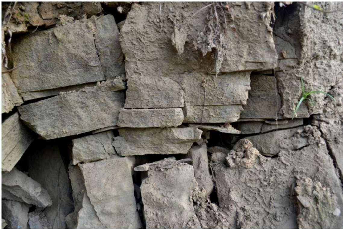
Plate 7.1.1.a Highly jointed and fractured sandstone
