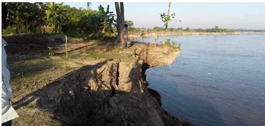
Plate 4.2: Land erosion at Bhogerpar by Brahmaputra River
