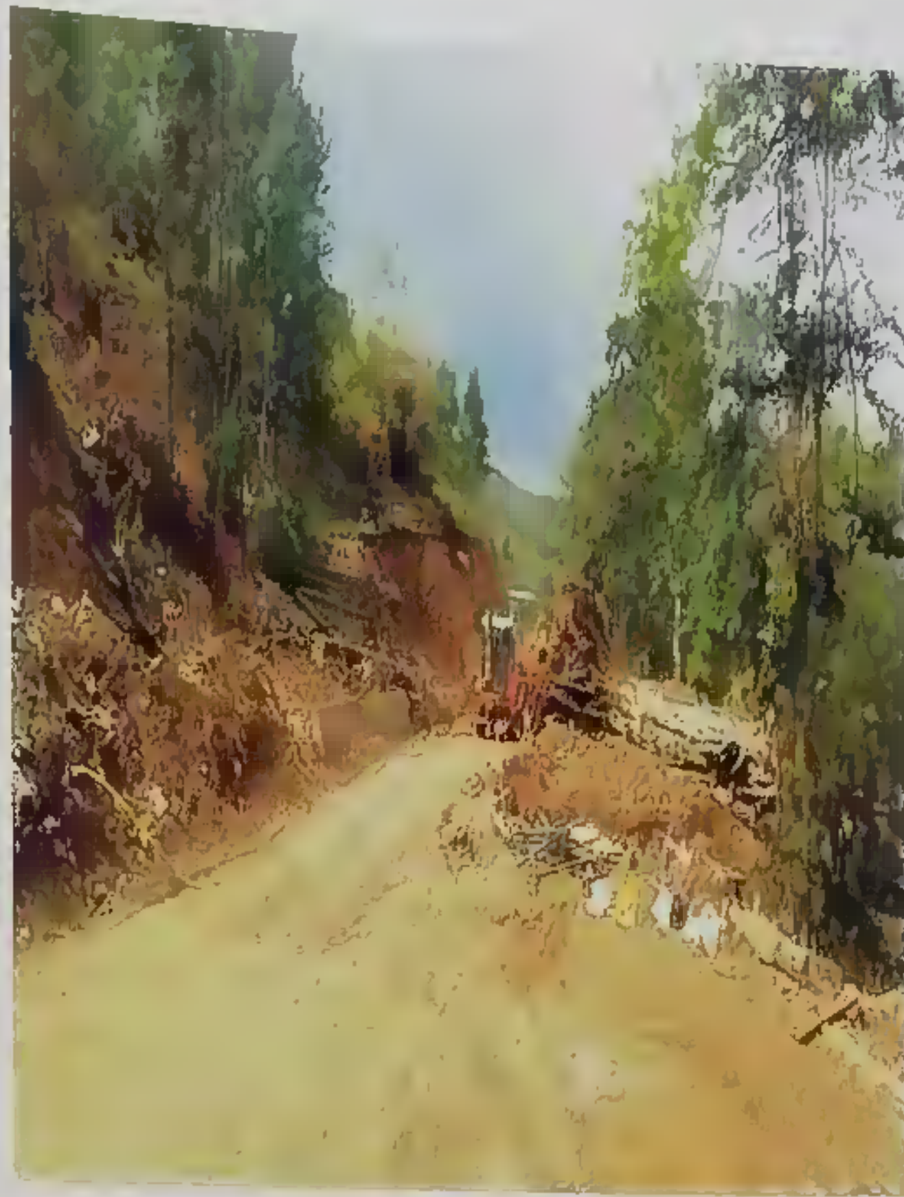
Plate : 4.15 Highway construction- a hazard to Environment
